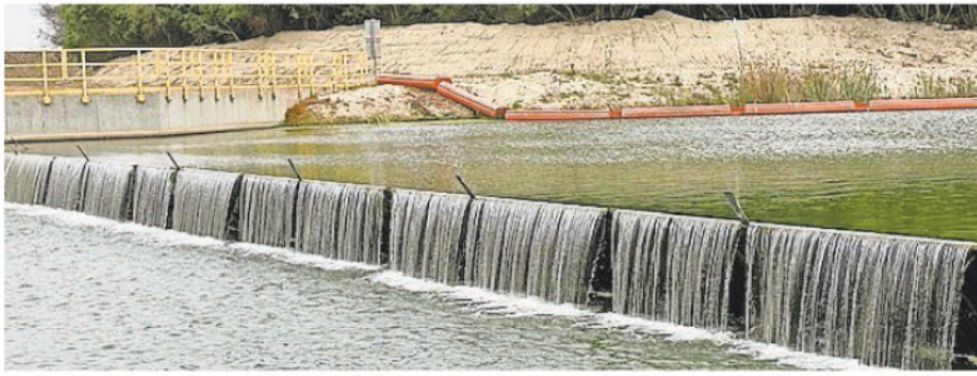
Salinas River Diversion Facility-Rubber Dam.
